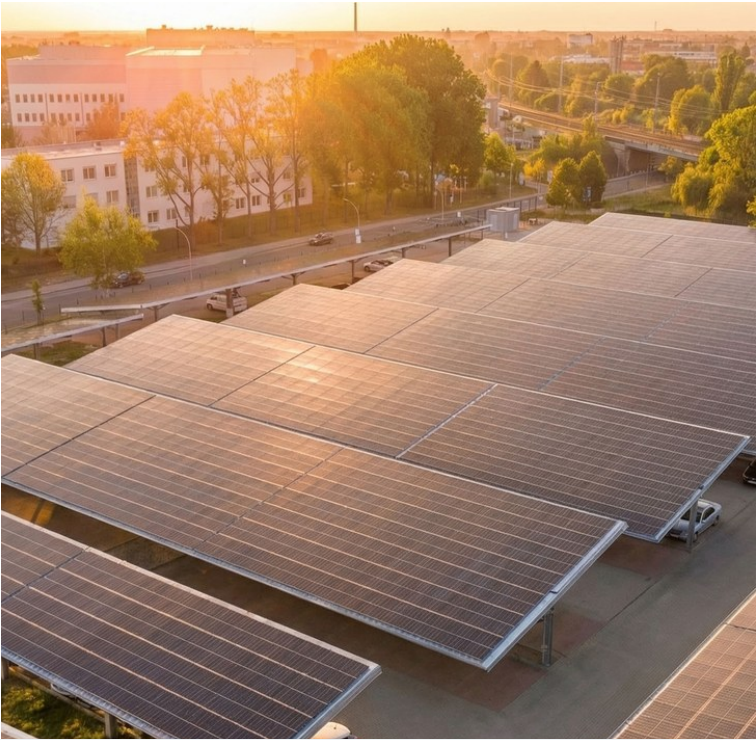
Through a newly installed photovoltaic system at our site in Oranienburg, Germany, we are generating enough renewable electricity to eliminate 650 tons of CO 2 emissions annually, approximately a 9% reduction in the site's total emissions.
