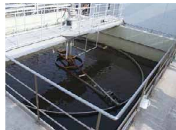
最新の生物処理設備 State-of-the-art biological treatment facilities
