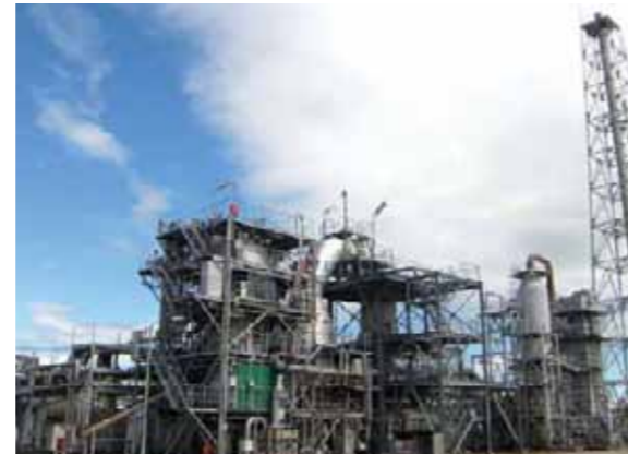
高COD廃液焼却設備 High-COD effluent incinerator
