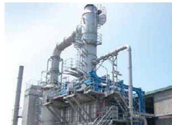
可燃物焼却設備 Combustible waste incinerator
